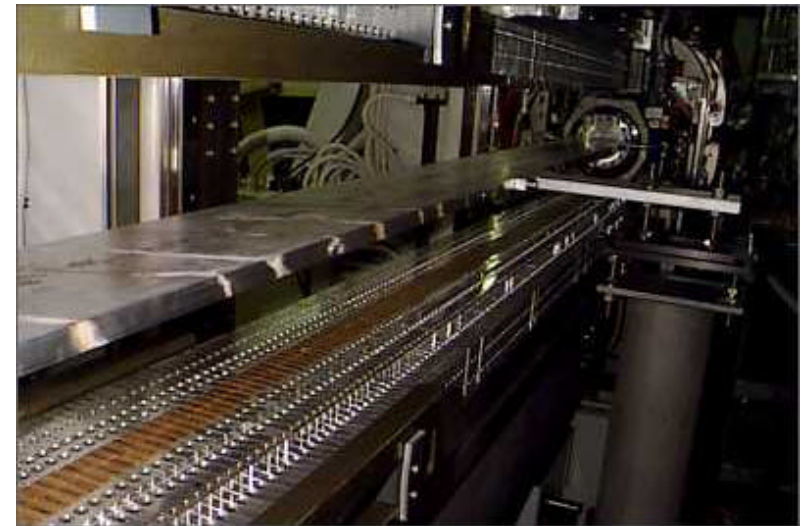
Elettra permanent magnet ID
